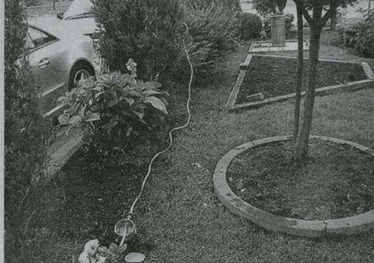
An investigator's photo shows the dangerous landscape lighting installation that led to one man's death.
